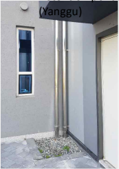
Infiltration by rainwater down spout in Incheon(Incheon)
